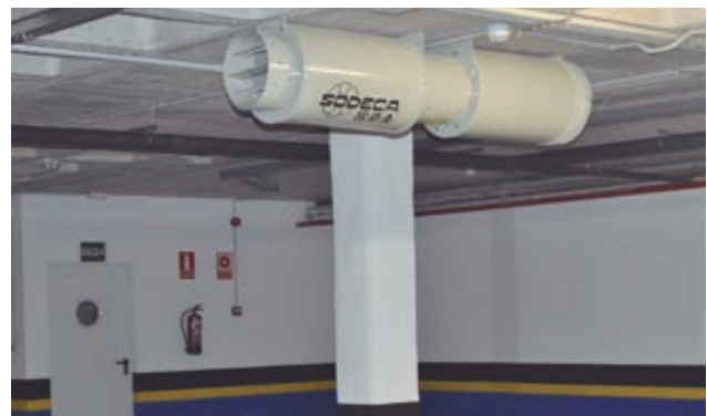
THT/IMP instalado en parking
